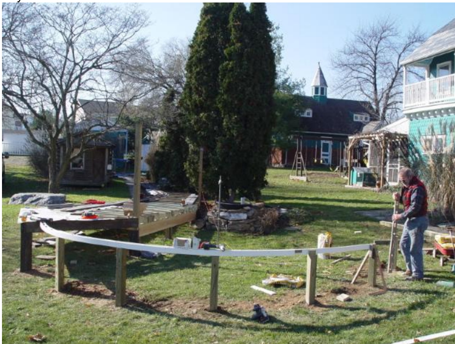
Twenty-four post holes and counting. Thanks to a lot of help, we're now 40ft from a complete loop!
